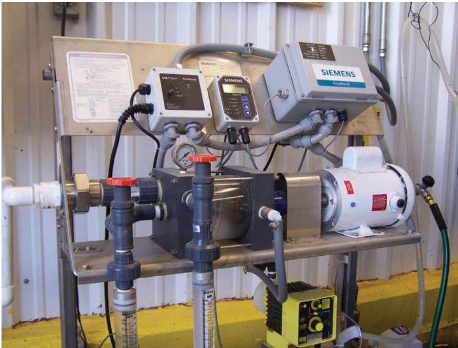
The enclosed part of the building housing the centrifuge and polymer feed is a 1000 sq. ft. building.
